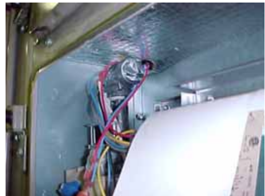
FIGURE 7 - Wiring from Gas Section Going to Blower Section
