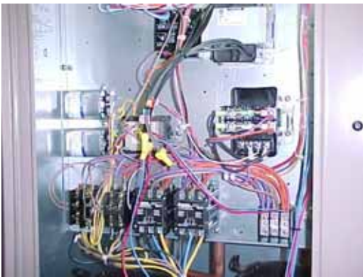
FIGURE 17 - Control Box View
